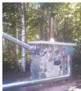
Outside stone furnace uses a small barrel stove as the firebox. Insulated air ducts pull warm air out and bring cool air back.
